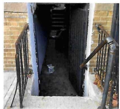
d. Basement stairway threshold at sidewalk level
