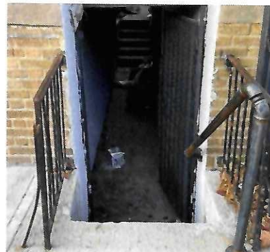
d. Basement stairway threshold at sidewalk level
